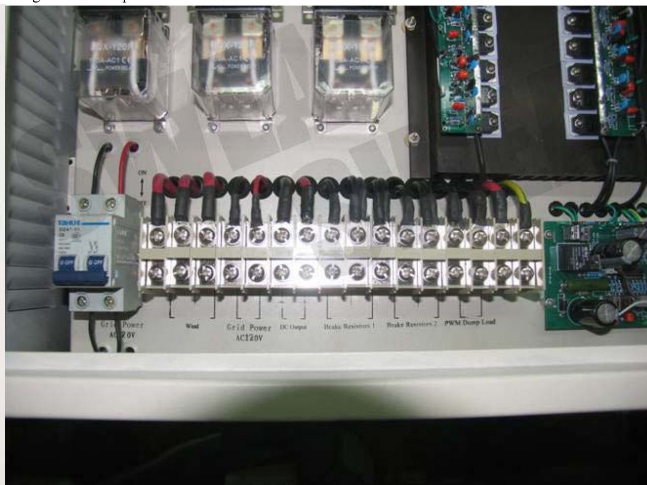
P7. Control Panel Connections
